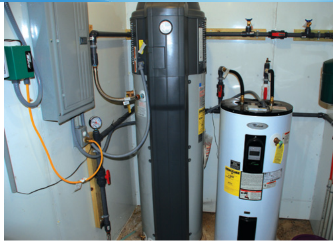
Figure 6. An electric heat pump and bulk storage tank in a mechanical room/closet. Used for radiant floor heating of a shrimp room.
