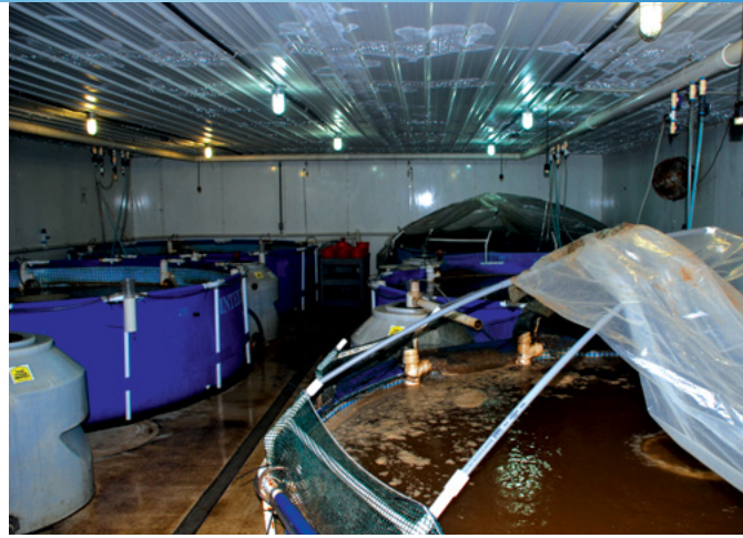
Figure 5. Patchy condensation on the ceiling of a shrimp production facility. Plastic covers on tanks retain heat and moisture within tank environs.
