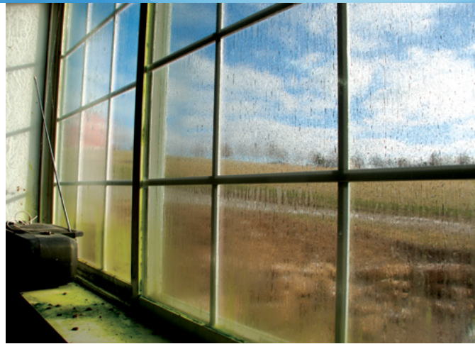
Figure 4. Condensation on the window of a tilapia production barn. Note the algal growth on the left side of the window.
