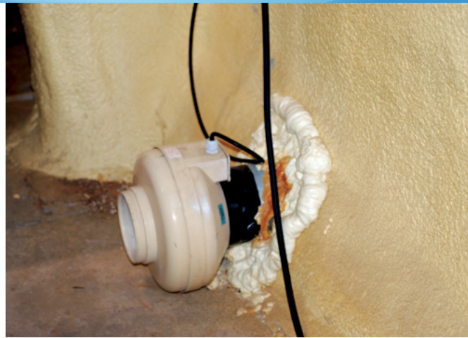
Figure 3. An electric exhaust fan for ventilation. Note the spray-on closed cell foam on the wall.
