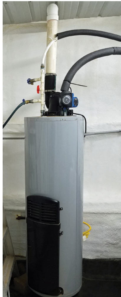
Figure 7. A household water heater with a circulation pump which also has a timer so it can be operated for a set period of time each day. The water travels to coils of polyethylene (PEX) pipe in each shrimp tank, then back to the water heater.
