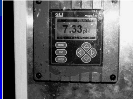
Controls Degassing of CO 2
