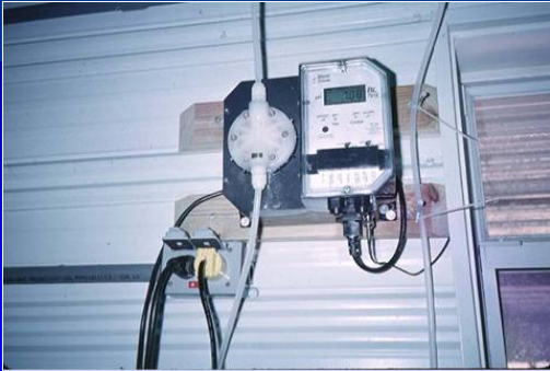
Control Dosing for pH Control
