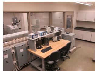
High Power Testing Bay
