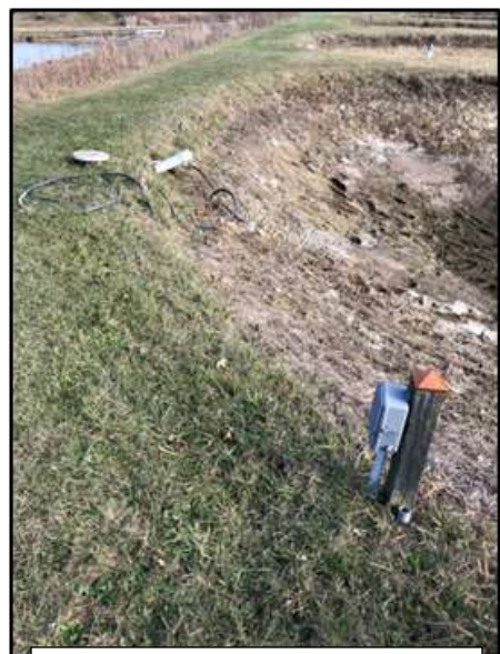
Electric and aeration lines at production ponds
